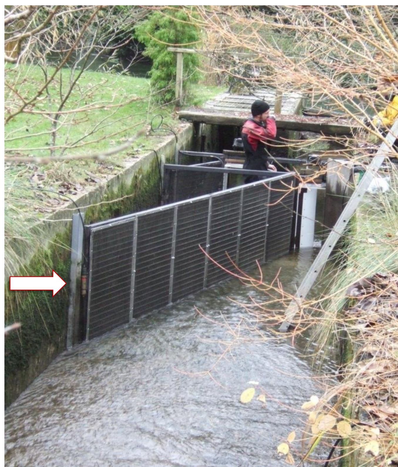
FIGURE 1 Image of the screen installation and bypass (to right and downstream of the screen) with hydrophones in place (flow direction is going away from the camera). Note the channel has been de-watered; experimental water levels are indicated by the high water line on the bypass deflector behind the ladder. Hydrophone H3 is indicated by the white arrow.
